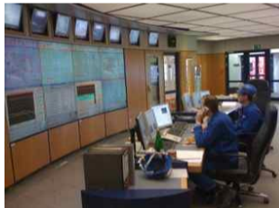
The control room of MVR, a facility considered by the European Union (EU) as the example of "best available technology" for waste treatment and recovery.
